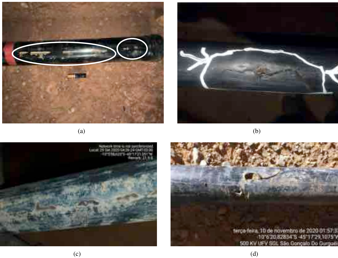
Fig. 5. MV cable attacked by termites..
